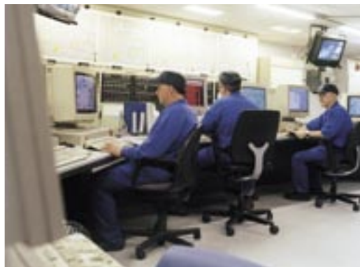
Remote operation from a central control room.
